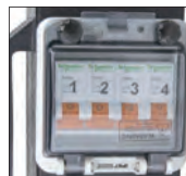
Each output is MCB protected.
